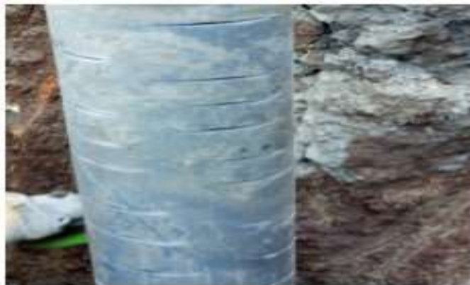
Figure 2f: PVC Pipe with perforations
