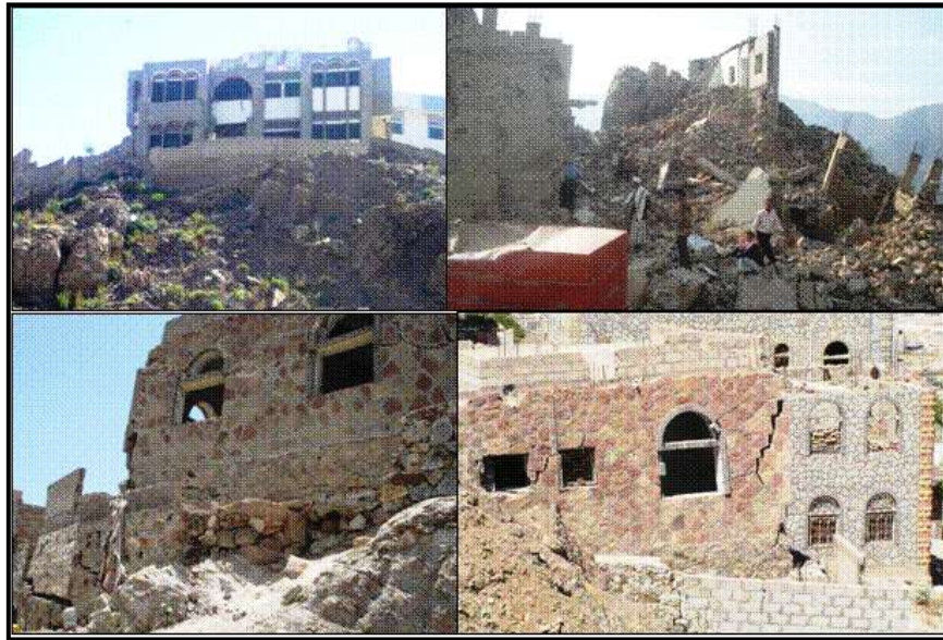
Fig.1. Photographs showing dilapidated conditions of buildings underlain by Tertiary volcaniclastics in the study area.
