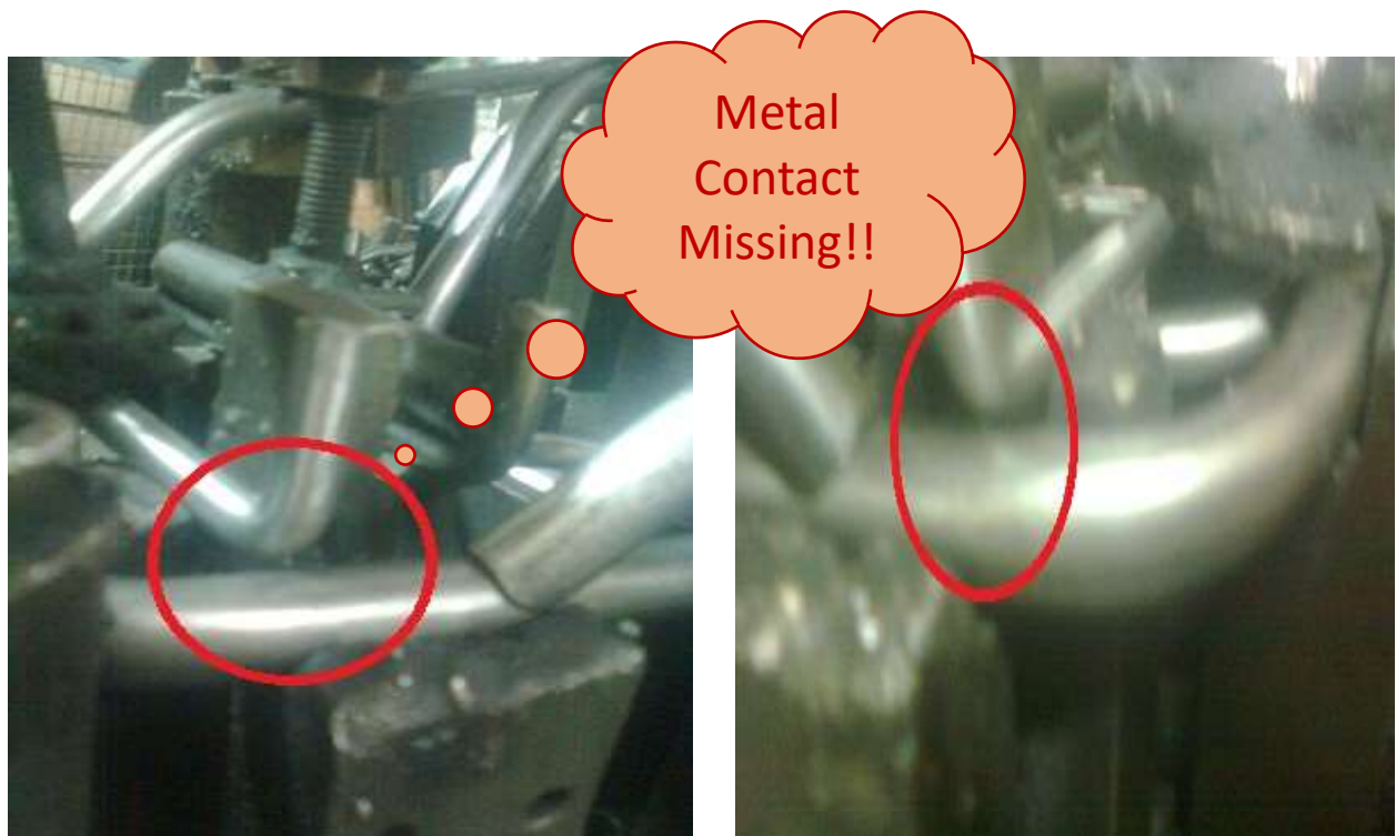
Figure 6 Gaps in welding fixtures
