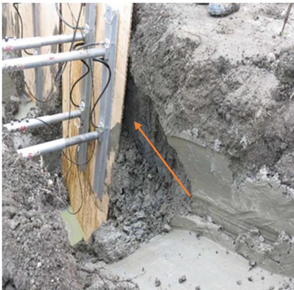
(c) Spotted soil cave-in to the trench after the installation of shoring system
