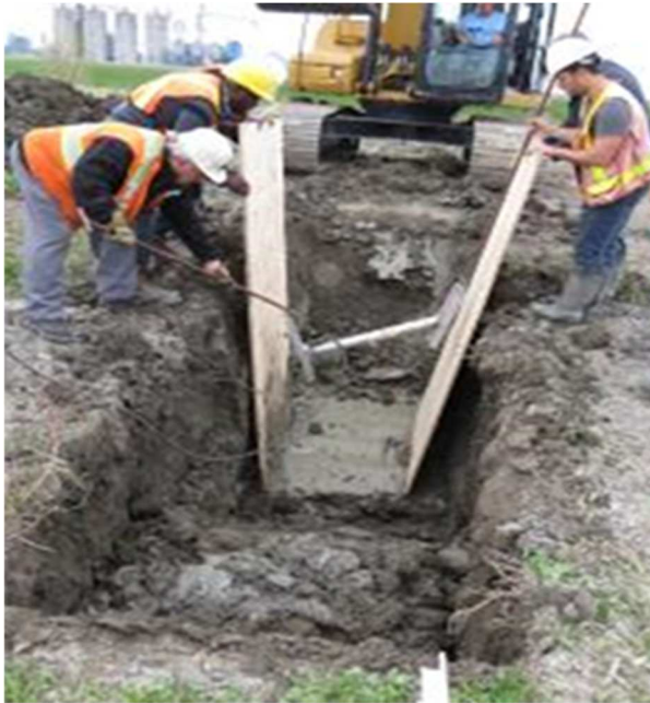
(a) Many people are required to installed this shoring system in this soft and sensitive clay.
