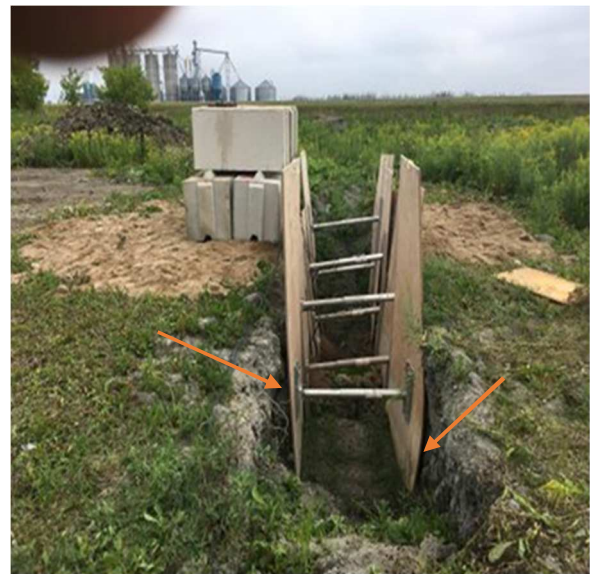
(d) Rain water washed away the soil between the plywood and shorowing soil.
