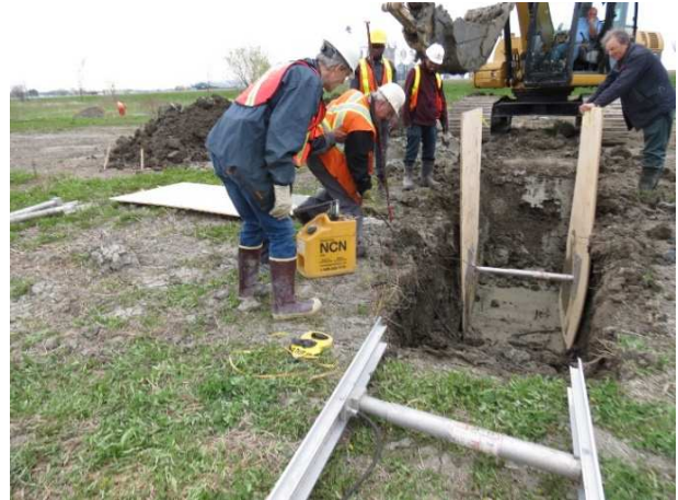
(b) Props of hydraulic shoring are placing and Hydraulic liquid is pumping to pre stress in the hydraulic cylinder.
