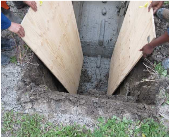
(a) Quick placing of plywood of hydraulic shoring system after right away the excavation
