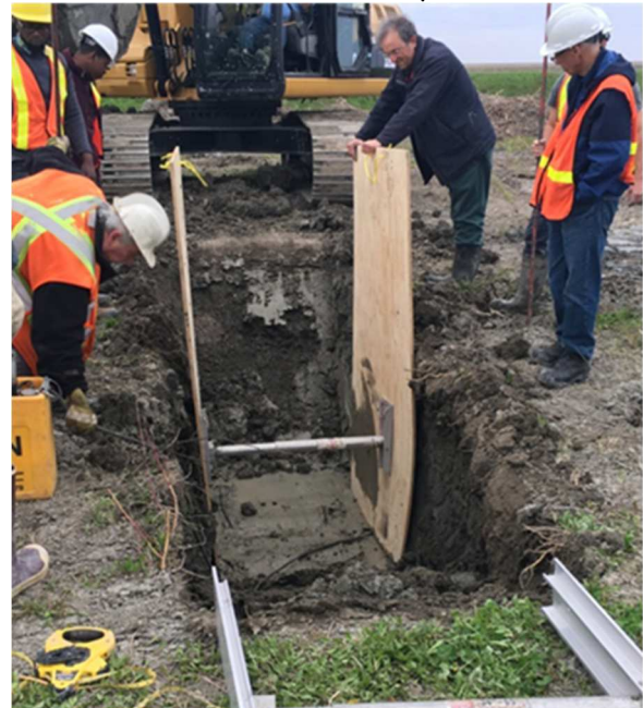
(b) It takes time and manpower to arrange the shoring in this type of soil.
